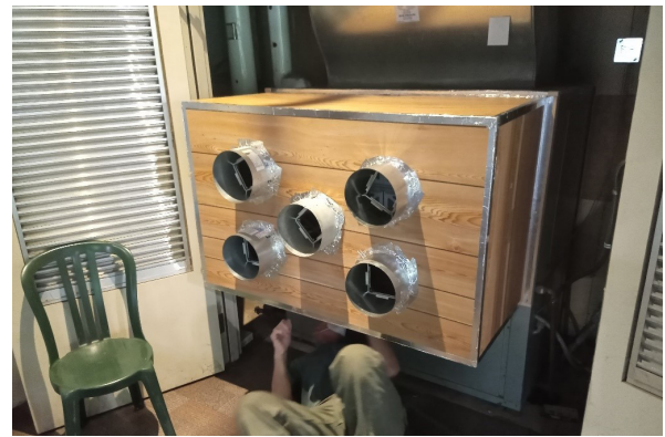
Figure 5. As part of the diagnostic monitoring, a custom airflow monitoring set-up was used by the EBCx team to check the operating parameters of the GSHPs.
