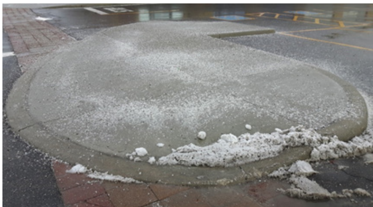
Figure 7 An example of an over-salted "orphaned" walkway
