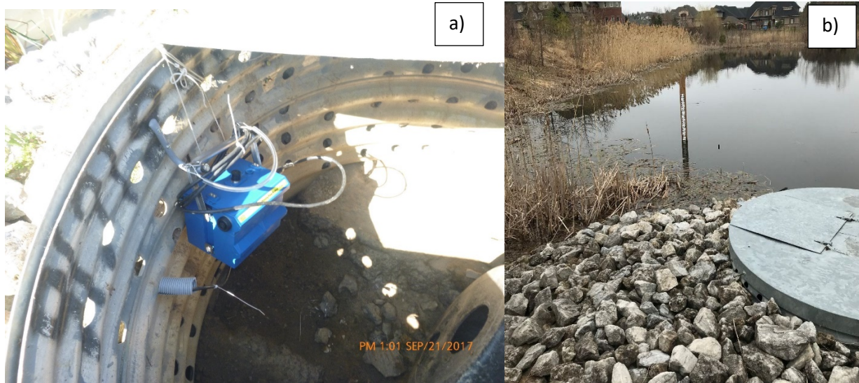
Figure D6: Shows how pond level measurements were taken. a) Shows ISCO level logger installed in the outlet structure, the cable to the sensor can be seen going into a grey plastic pipe that leads out to the pond. b) Shows the location of the staff gauge, which was used to calibrate the level sensor. The small piece of rebar in the water beside the stage indicates the location that the level sensor was installed within the pond.
