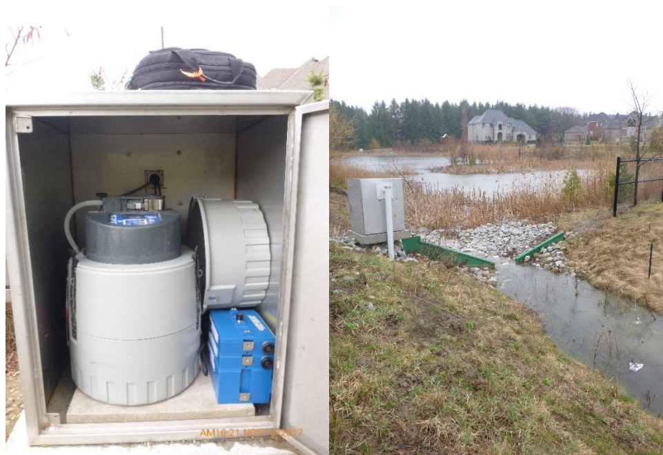
Figure 7: Typical monitoring equipment installed at Pond A monitoring stations
