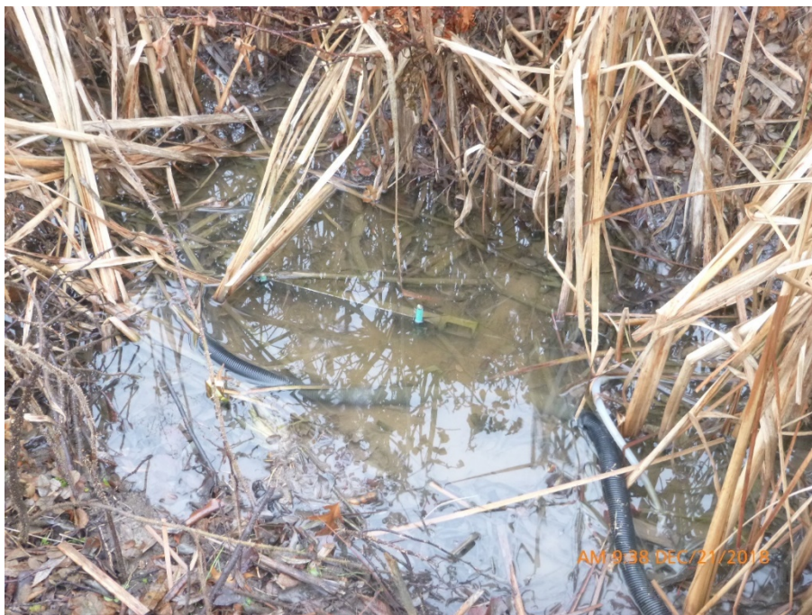
Figure D8: Shows how turbidity sensors were installed in the inlet swales. Sensors were installed upstream of other instrumentation (sampler intake/ conductivity sensor) to minimize disturbance. Rebar was used to secure a metal plate, and the sensors attached to the plate using u-bolts to keep the sensors secure during high flow, but to also allow for easy removal for cleaning and maintenance
