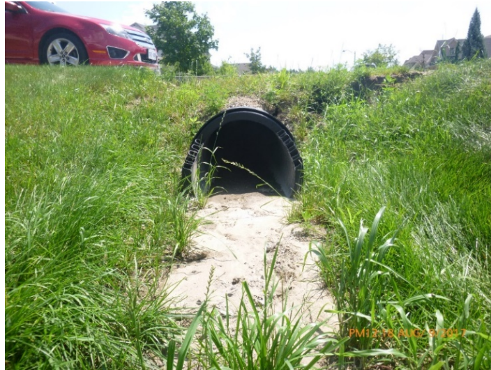
Figure 21: Culvert and grass swale with accumulated sediment in it.
