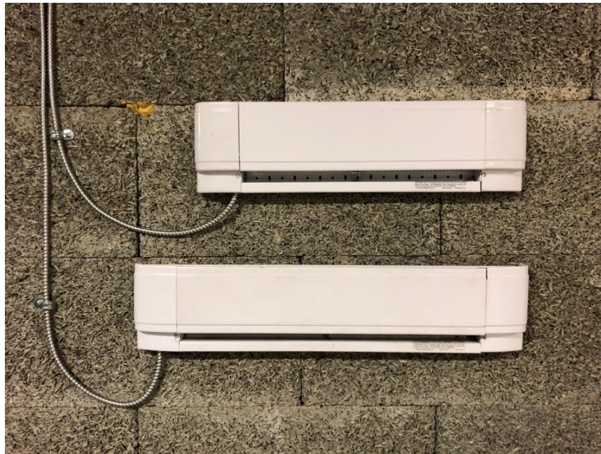
Figure 5-5. Auxiliary loads were electric resistance heaters.
