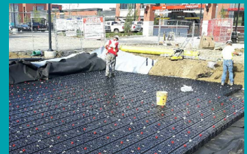
Figure 3: Infiltration Chamber and Stormwater Re-use
