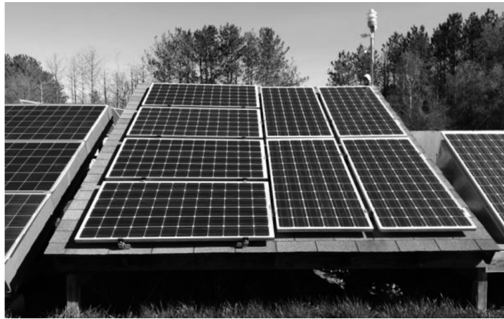
Figure 2. Eight modules were mounted on a roof-section.
