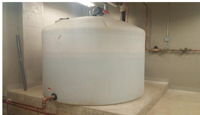
Figure 3. Rainwater tank at CVC
