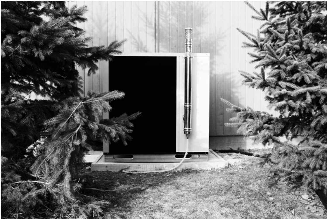
Figure 1. The gas absorption heat pump installed outdoors on a concrete pad at the ASH Lab
