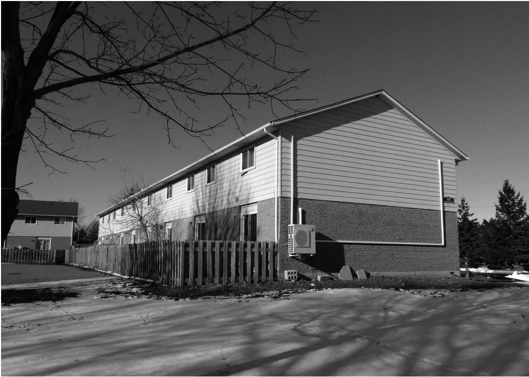
Figure 2. Outdoor refrigerant lines connecting condenser and indoor fan coils
