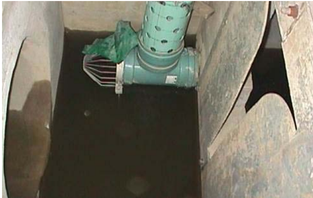
Figure 11: Orifice control pipe within the outlet control chamber for baseflow augmentation (Markham, ON)
