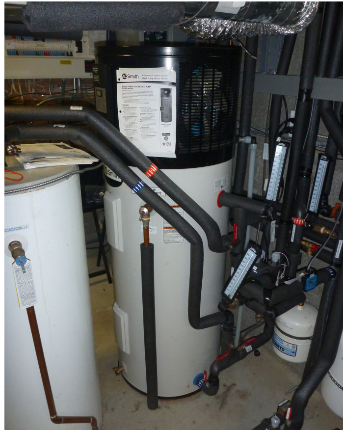
Figure 2. The A.O.Smith ASHPWH installed in the basement of the test site.
