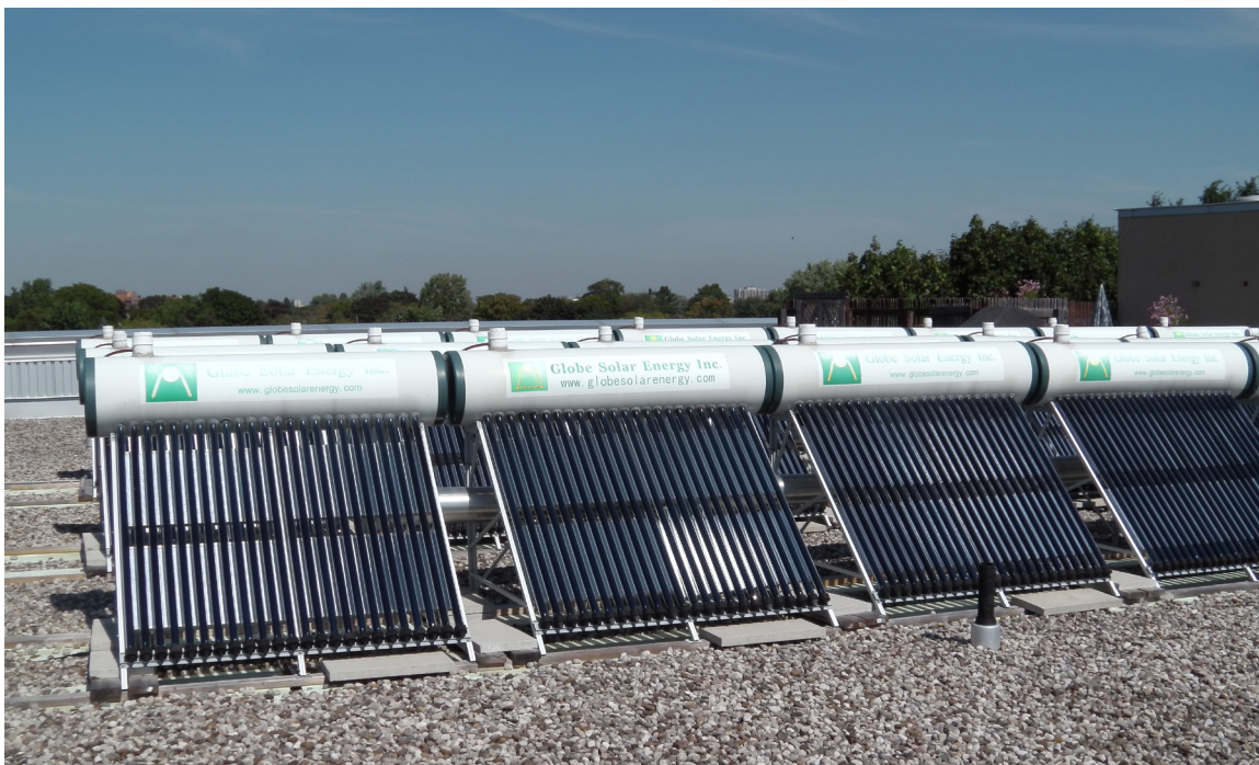
Wilmar Court evacuated tube solar water heating system, Toronto, ON
