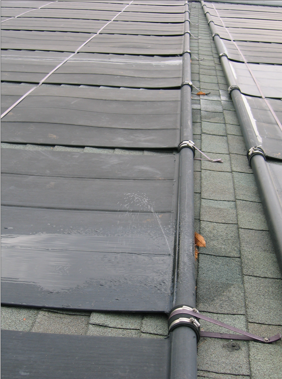
Figure 6. Two leaking solar collectors.
