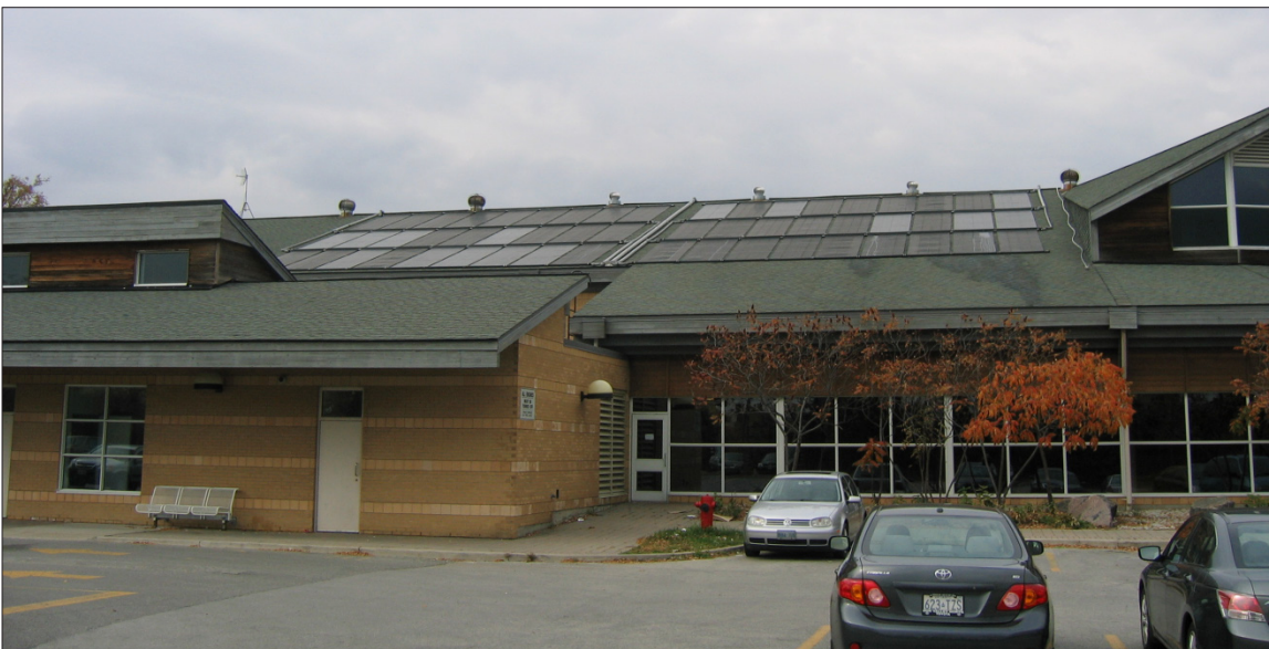
Figure 4. System view picture taken in Oct, 2010 showing collectors that had been replaced up to that time. The new collectors appear gray on the picture. The collectors have now all been replaced and the system should have normal operation n 2012.
