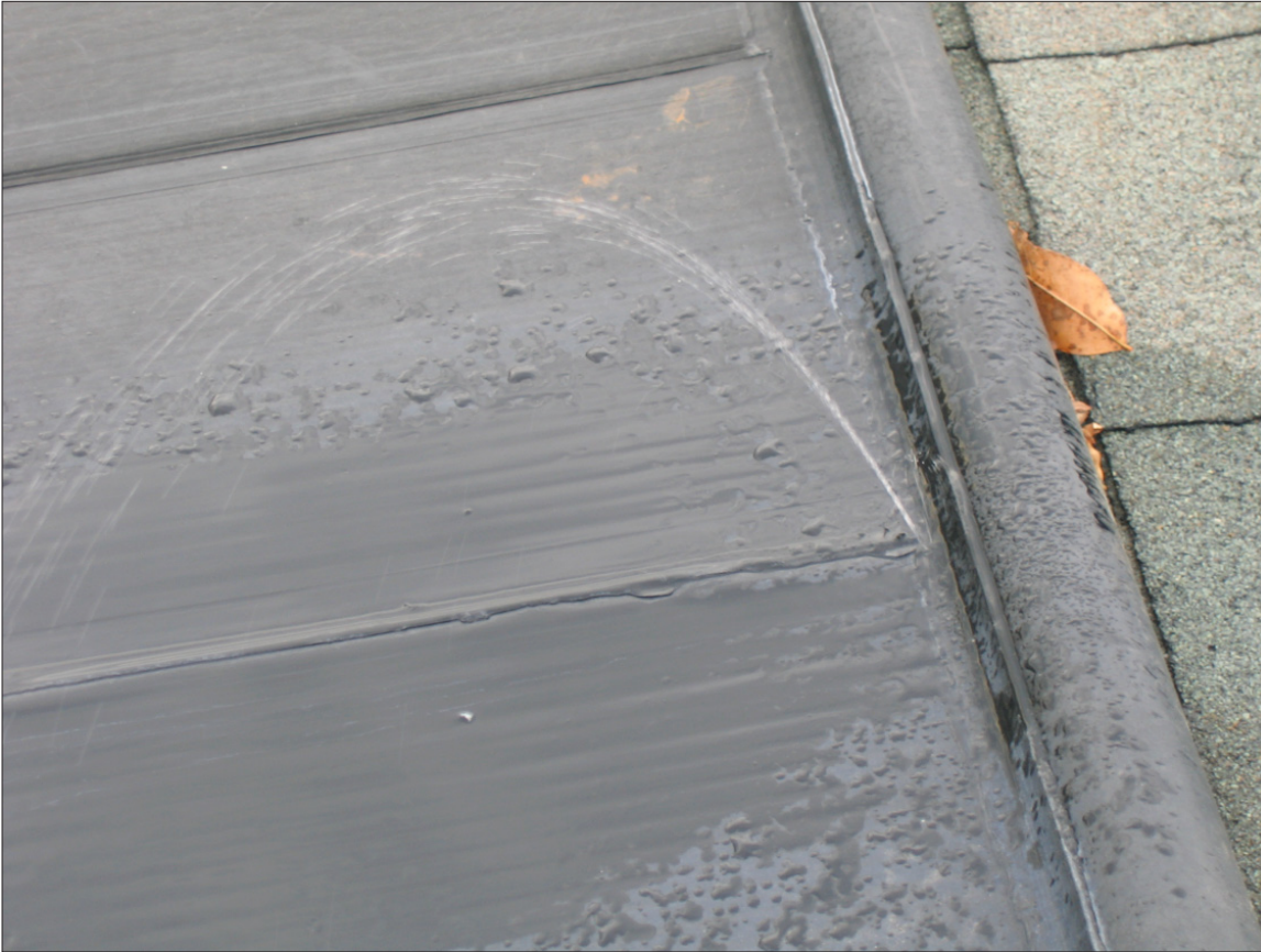
Figure 3. Solar collector with leakage at the plate/header welding.
