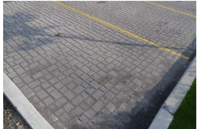
Figure 6. Sediment build-up and clogging in the permeable pavement
