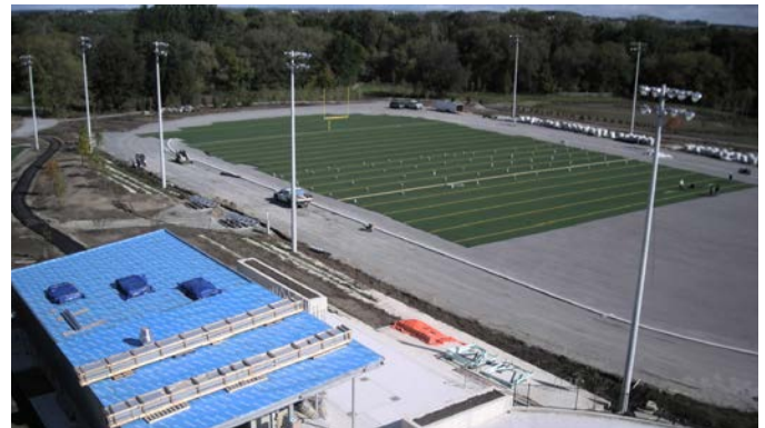
Figure 3. Cistern placement during construction (above); artificial field above cistern (Pictures courtesy of Schollen and Company Inc.)
