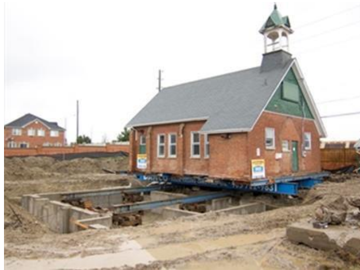
Figure 4.61: Ebenezer Community Hall in the process of getting moved back from the road. 63
