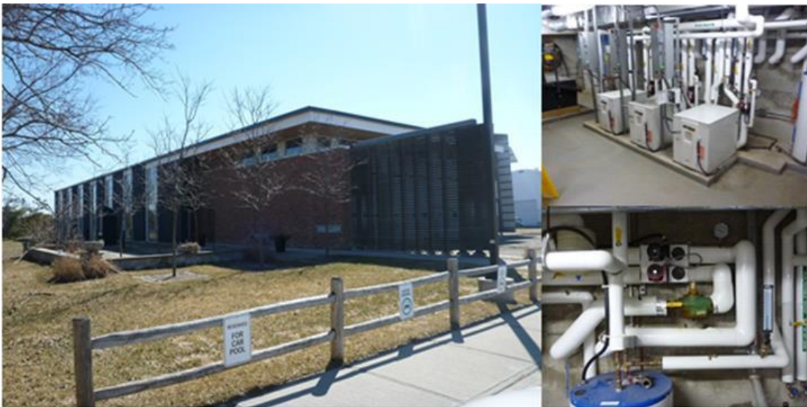
Figure 4.24: (Left) The Restoration Services Building exterior. (Top right) The three ground source heat pumps power the geoexchange system. (Bottom right) Ground loop pumps.
