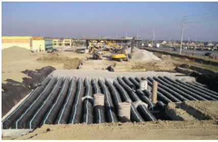
A stormwater infiltration chamber system being installed on silty to clayey glacial till soil that is common in the Greater Toronto bioregion.
