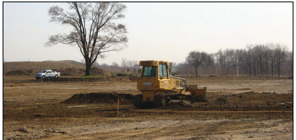
Topsoil being reapplied during construction (foreground) and a tree protection zone (background).
