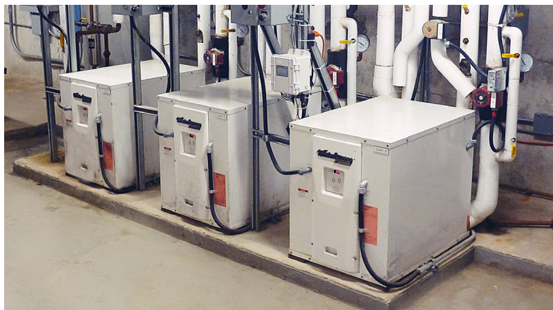
Figure 1. Three water-to-water heat pumps in the basement mechanical room of the Restoration Services Centre facility.
