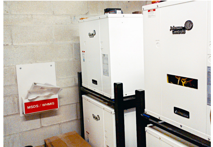
Figure 1. Four geothermal heat pumps in the North Fire Hall.
