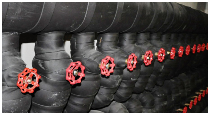
Figure 1. Ground loop manifold in basement parking garage of GreenLife Condominium.
