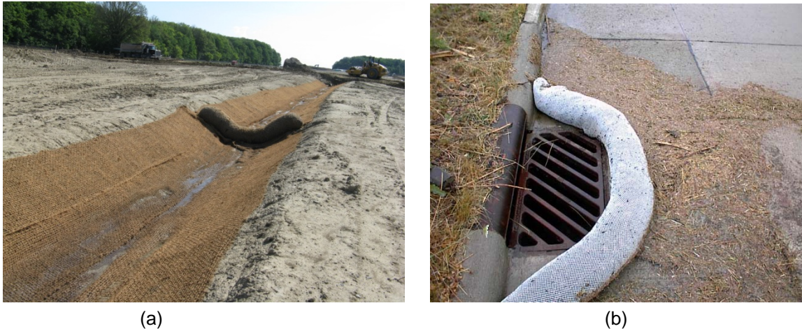
Figure 3.1: (a) cut-off swale installed during earthworks and (b) storm drain inlet protection installed for underground services/building construction ( Note: control shown in (b) is not installed at study site )
