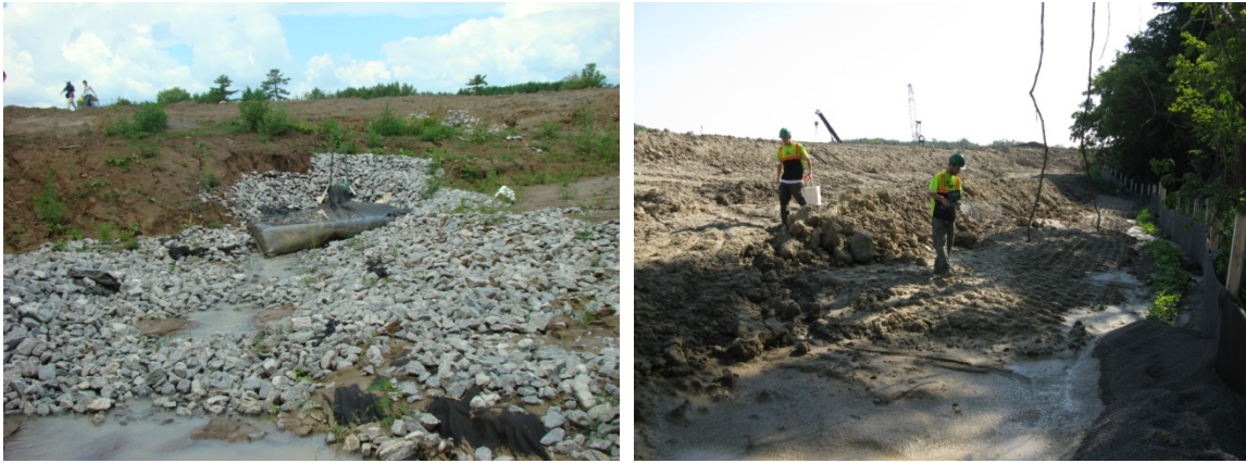
Figure 2.4a: Pond 2 outlet scour pool and surrounding slopes before stabilization.
