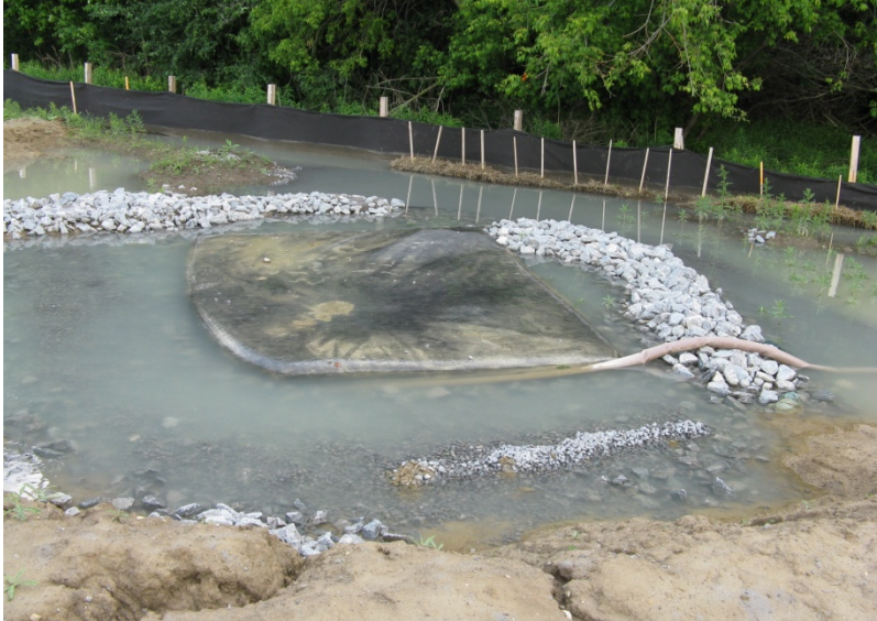
Figure 2.9: Sediment bag and scour pool used for pumping down pond 1 during spring 2008
