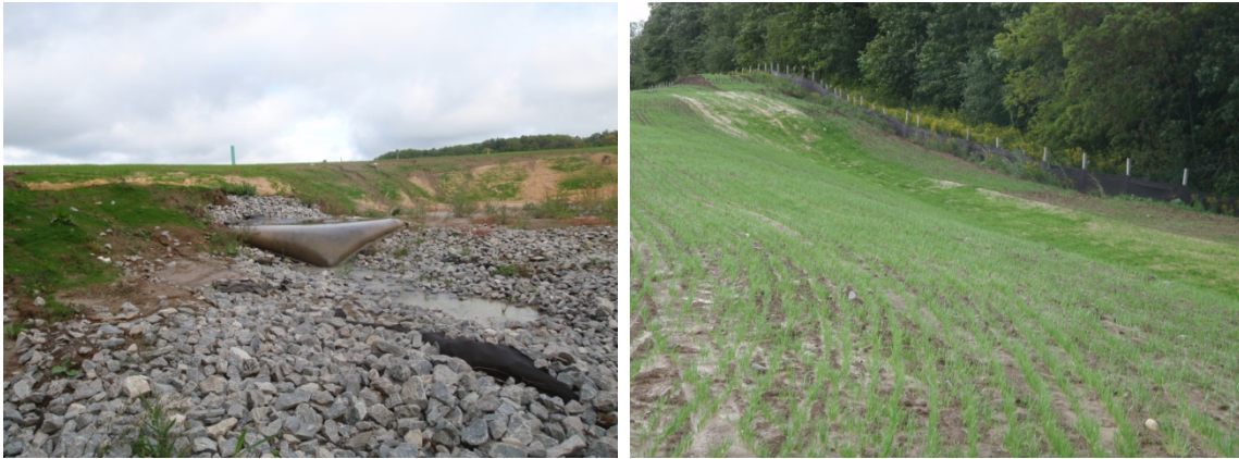
Figure 2.4b: Pond 2 outlet scour pool and surrounding slopes on September 14, 2008, after stabilization.
