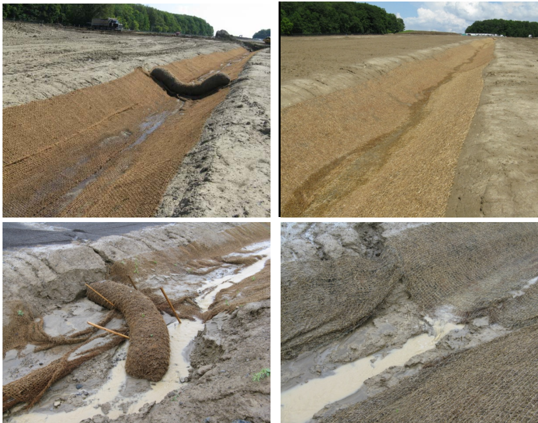
Figure 2.8: Coir matting and coir logs in a cut-off swale at the study site. Top images taken after installation in late June 2008 and bottom show their condition in late July 2008.
