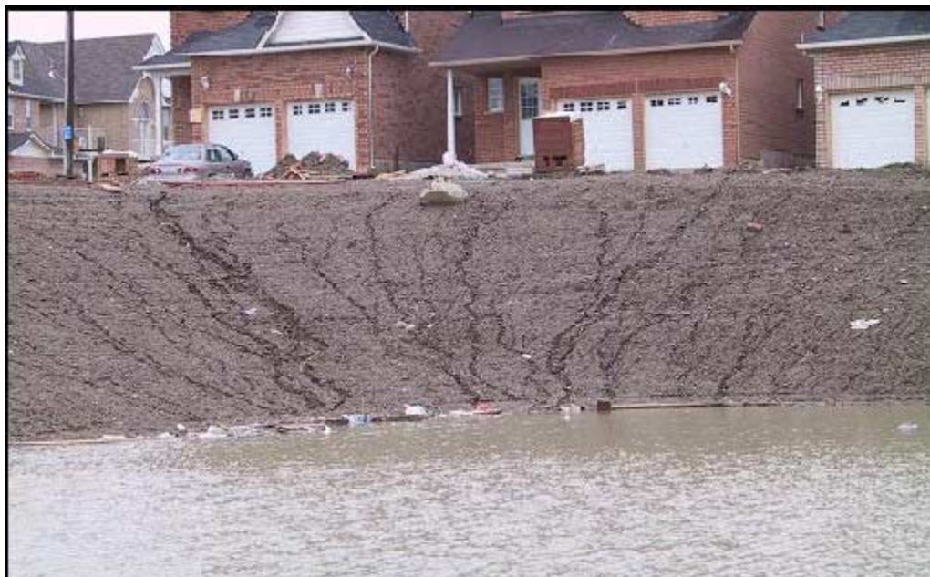
Figure 3: Ballymore pond bank erosion
