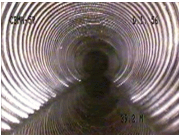
Figure 11a: A frame from the CCTV inspection of the MacFarlane system
