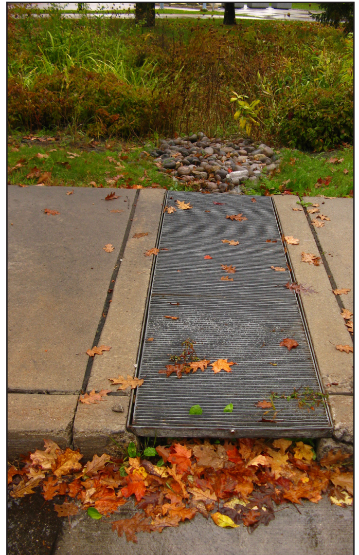
Figure 5. Leaves clogging inlet to bioretention
